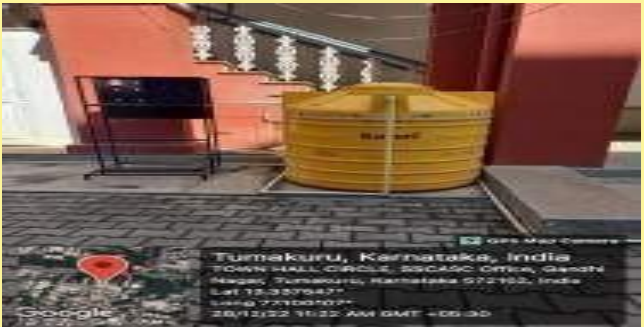
Over head tank for recycling the water
