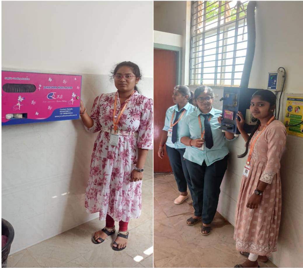
Sanitary Pad Vending Machine and Incinerator machine in the Ladies Wash Rooms
