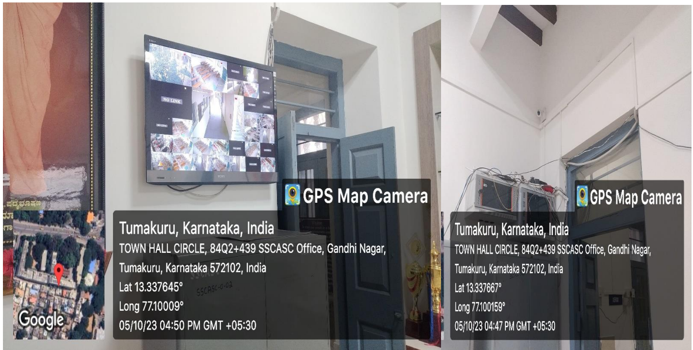
CCTV Camera surveillance and Monitor
